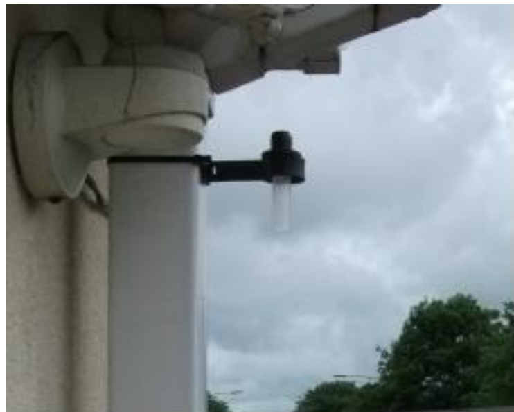
Use of a diffusion tube to monitor roadside NO2 levels from the façade of a property.
