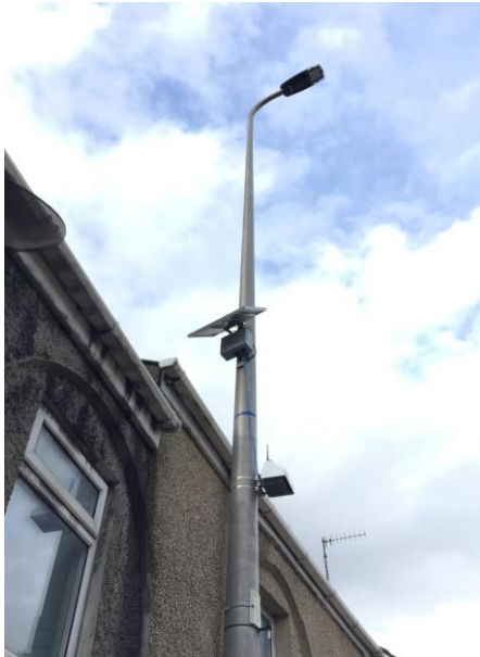
Use of an AQMesh Automatic Analyser to monitor road side Pollution levels.
