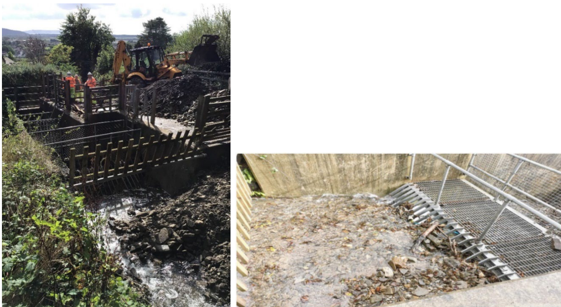
Figure 22 - Photos of the debris removed after the flooding event on the 4 th October 2021 at Cae Ffynnon.
