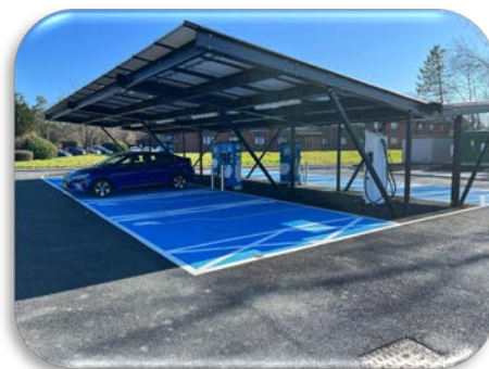
Our new, first of its kind in Wales, electric vehicle charging hub in Cross Hands
