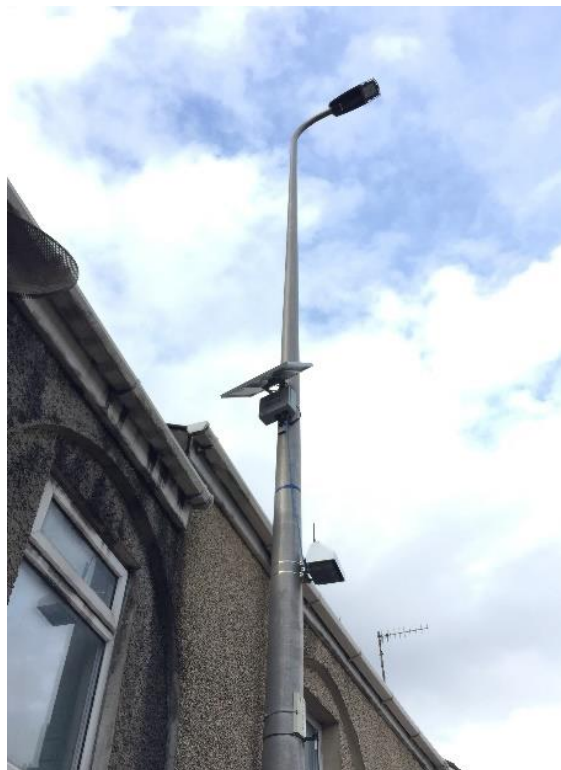
Use of a AQ mesh Automatic Analyser to monitor roadside pollution levels.
