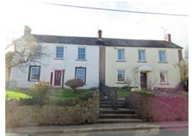
Rubble stone retaining wall to raised forecourts of 'Kieffe House' and 'The Kieffe'
